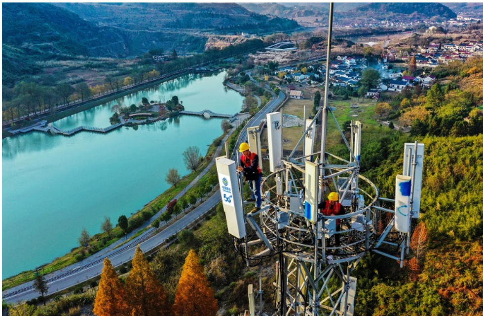
The 5G base station of China Mobile.
